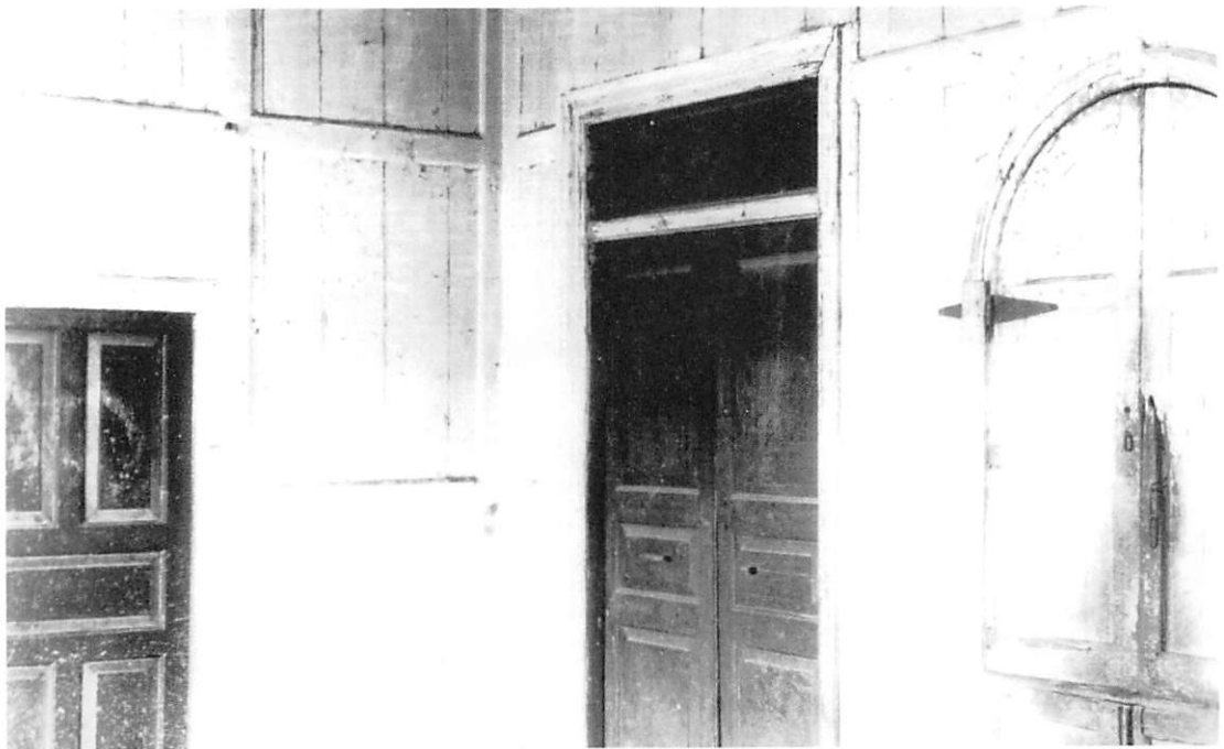
The interior walls are made of vertical boards affixed to the ceiling and floor. The horizontal boards were added to stabilize the vertical sheathing.
